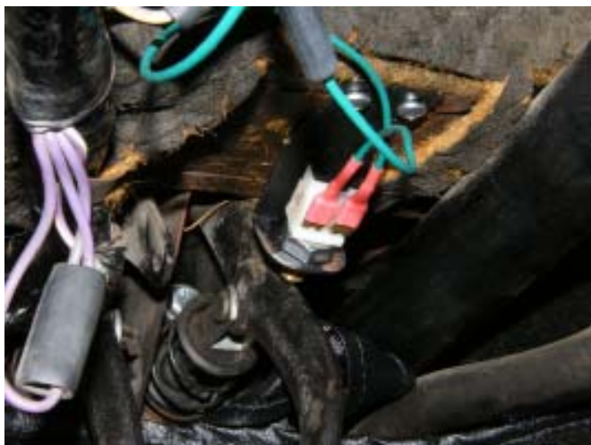
Figure 5. Here's the installed switch, again with the prototype switch.
