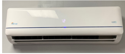
Indoor unit on the wall
