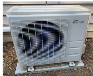
Outside compressor set
